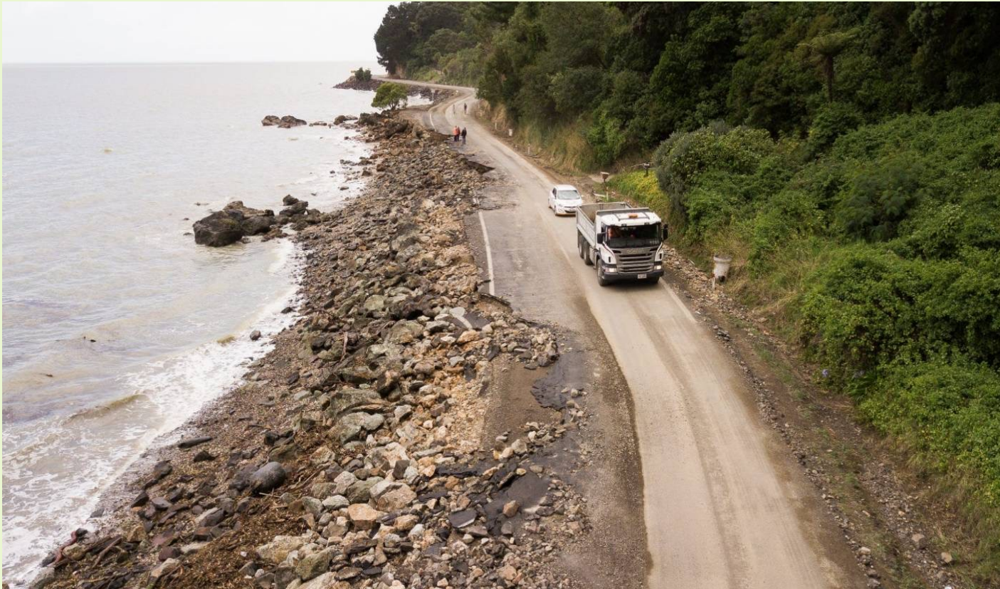
Thames Coast Road 2018 storm events
